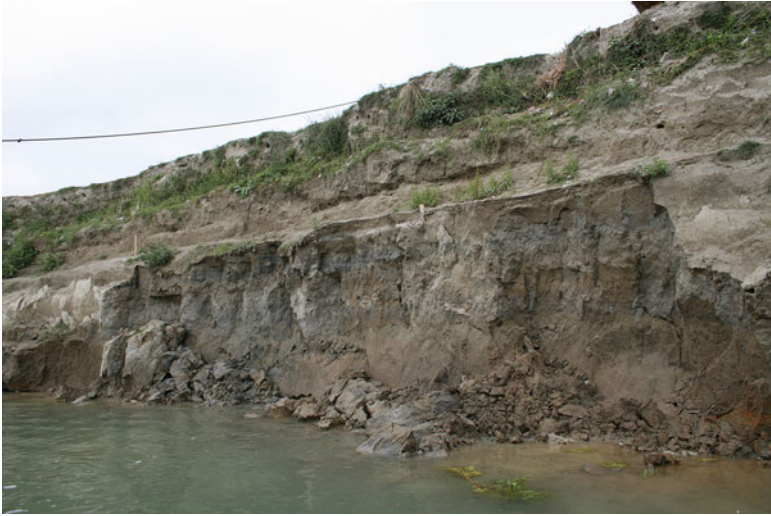
Photo 5.4 Bank erosion in Brahmaputra near Majuli Island, Jorhat district, Eastern Assam
