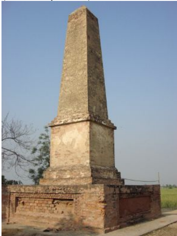
55. Sabraon monument in present day. A short, four-sided obelisk made of burnt brick, it is now in need of repair and attention.
