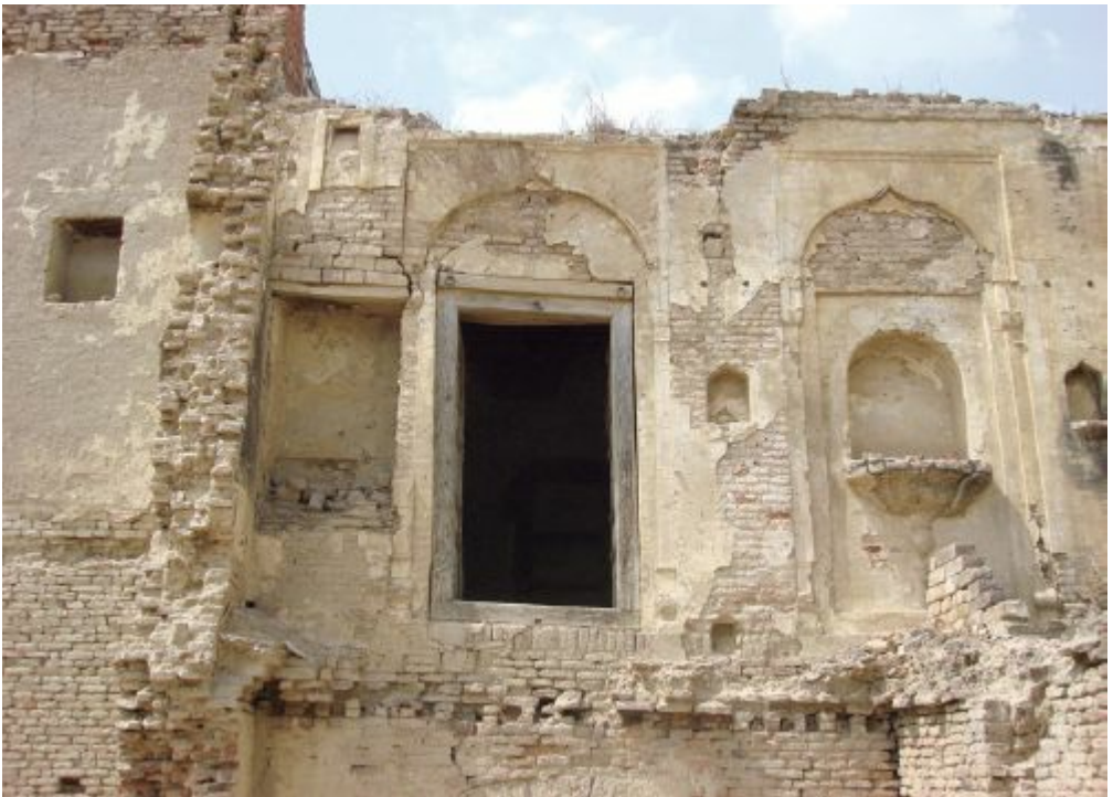
31. Exposed sections of the second floor of Mudki fort, revealing decorative work and construction.
