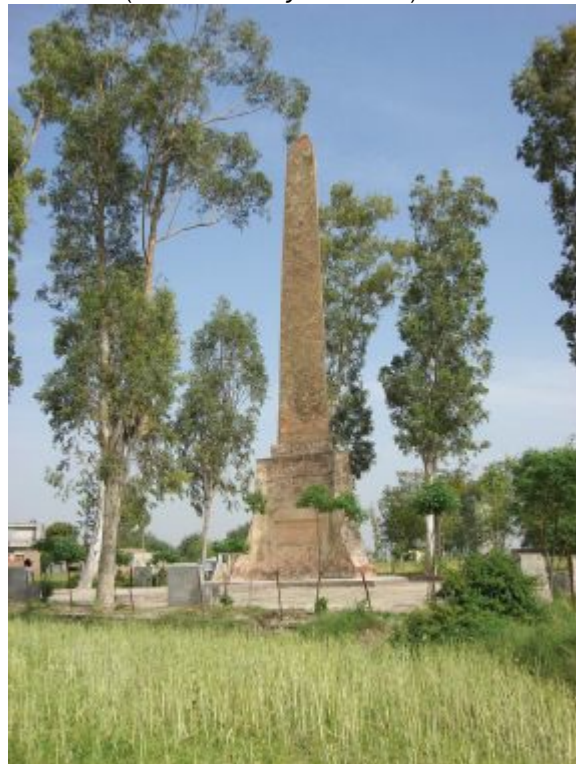
35. British monument at Ferozeshah in the present day. The structure remains in good condition, although the plaques that originally decorated it have disappeared.
